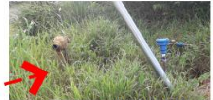
EXISTING FIRE HYDRANT WATER METER
